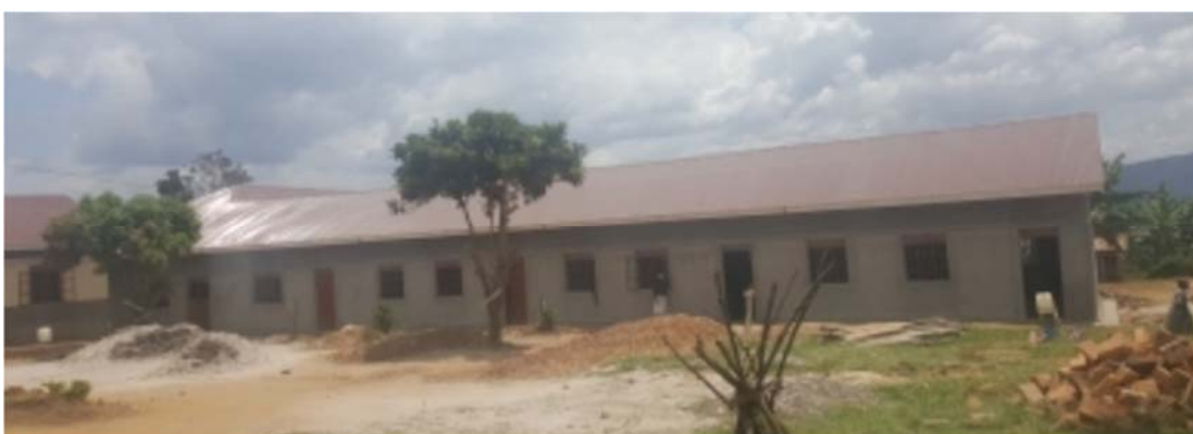
The Administration and Four Classroom Block nearing completion. The original condition of this block was worse than the Three Classroom Block
